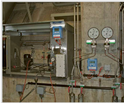
Fig. 6. AMI CACE in hotwell station.
